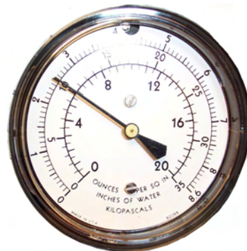
With tank valves closed, propane inlet line pressure must be reduced to 10” of water column for leak testing
