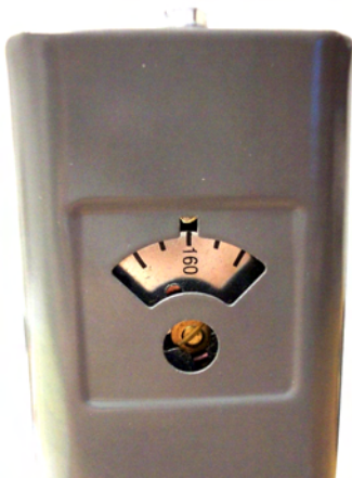
Operator Control – Set at 160°F for testing. Reset to 200°F for normal operation.
