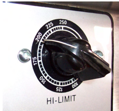
Hi-Limit Control – Set at 200°F for testing. Reset to 230°F for normal operation.
